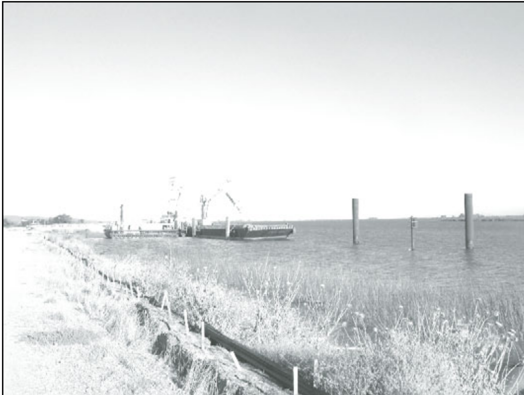
Machinery used in the privately funded Montezuma Wetlands restoration project in California (Photo by Levine-Fricke).
