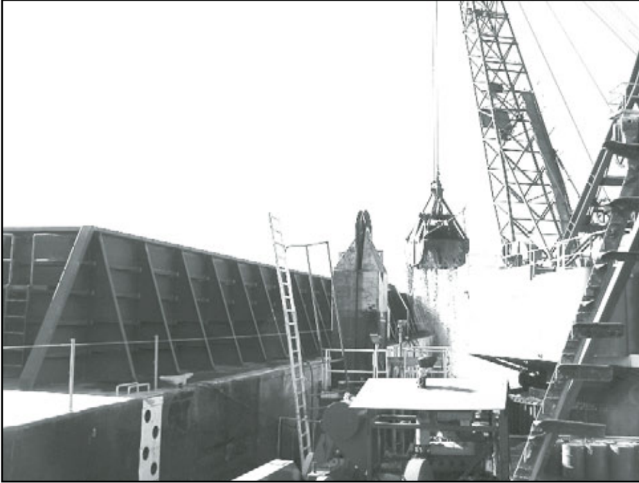
Dredging operations in Port of Oakland, California (Photo by Port of Oakland).
